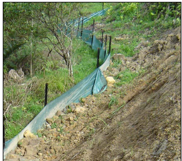
Getting the solution in place - Sediment controls installed on building site to retain sediment and prevent entry to stormwater drains or streams
