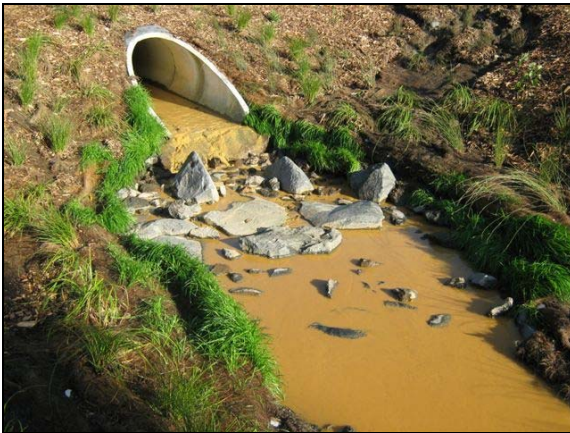
The problem - Sediment discharge from just three uncontrolled building sites into a once clean stream.
